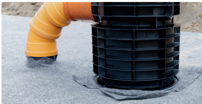
The geotextile is cut in and is pushed over the pipe adapter
