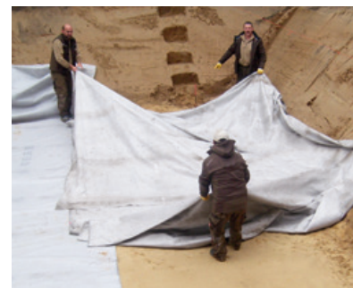
After creating a level surface which is free of stones, even and without gradient the trench is lined with a filter fleece.
