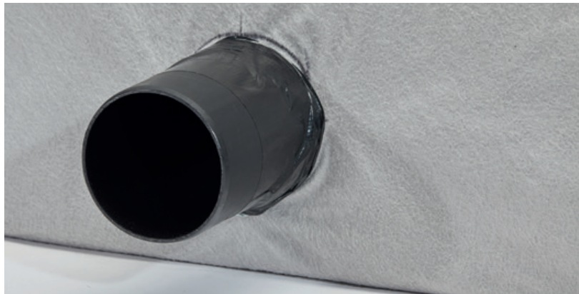
The geotextile is cut in and is pushed over the pipe adapter
